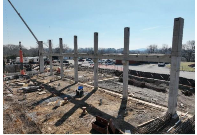
Bridge Crane Elevated Support Beam
